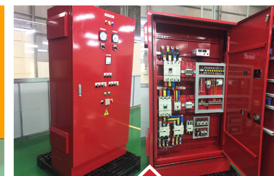
Fire Pump Control Panel
